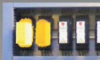
Thermal Fusion image of an overheated circuit breaker
