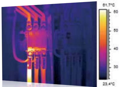
Infrared inspection reveals an overheated electrical connection that was discovered just in time to prevent a fire and possibly even save lives.
