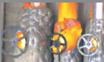
Thermal Fusion image of steam leaking from a pipe due to insufficient insulation
