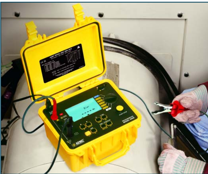
Model 5060 performing insulation test on a generator.
