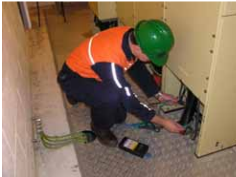
Figure 9: Cable screen measurement
